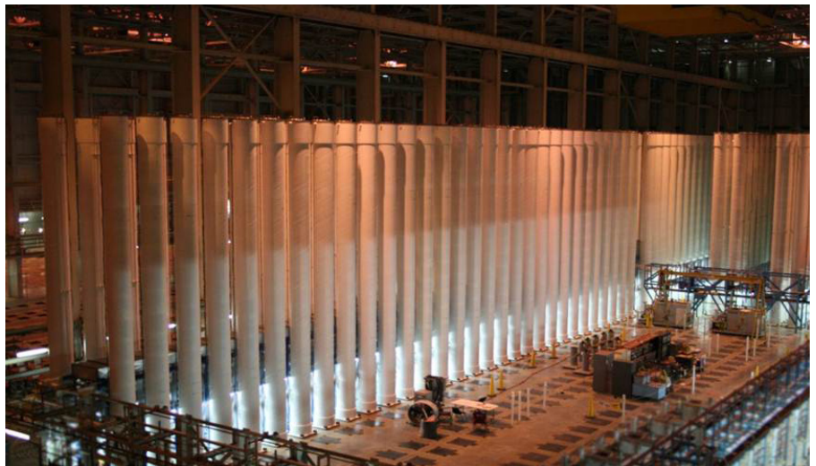
Gas centrifuges are typical dual use goods: they may be used to enrich uranium for civilian as well as military purposes. USEC
