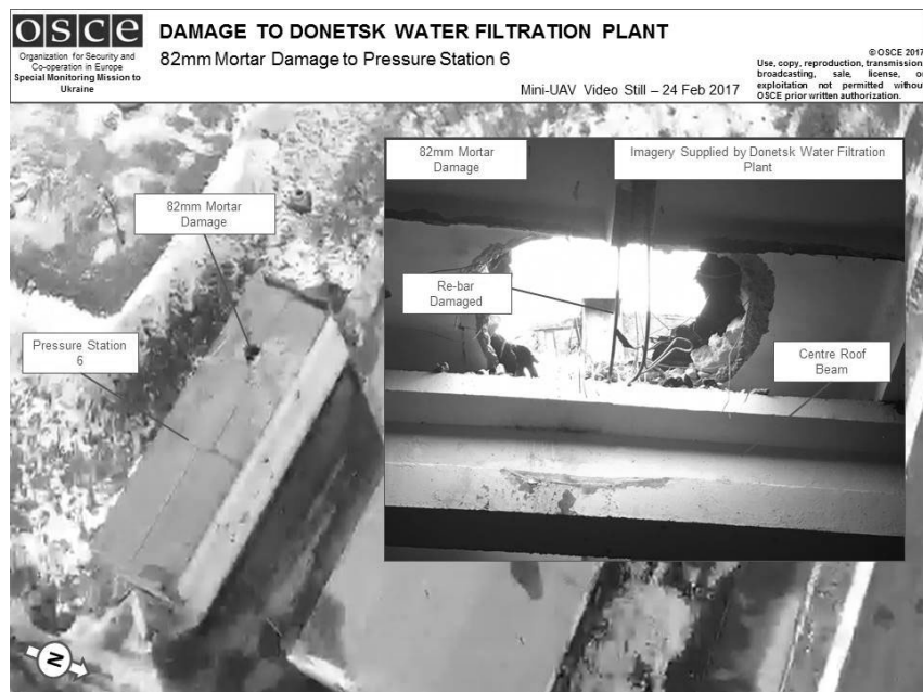
Figure 24: Monitoring of essential infrastructure. Impact site assessment at the Donetsk Water Filtration Station
