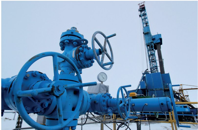
Valves near a drilling rig, operated by Gazprom, at Bovanenkov gas field on the Arctic Yamal peninsula, May 21, 2019. Maxim Shemetov / Reuters
