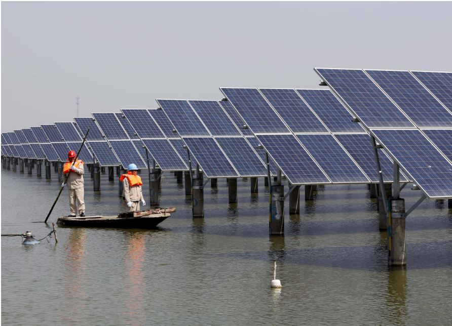
Employees row a boat as they examine solar panel boards at a pond in Lianyungang, Jiangsu Province, China. China Stringer Network / Reuters
